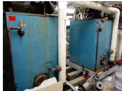
Defunct Burnham Boilers
