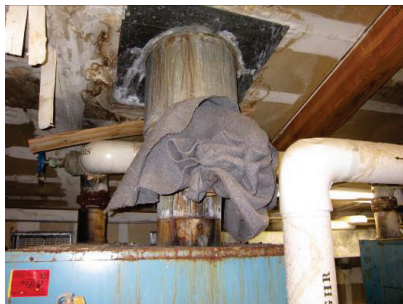
Blocked Boiler Stack and Ceiling Deterioration
