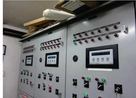
Generator Control Panels
