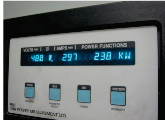
Power Control Panel
